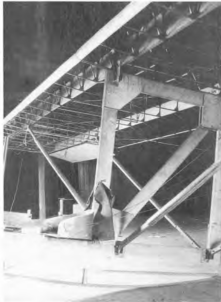
First assembly of the SGP 1-1 in the barn loft.
